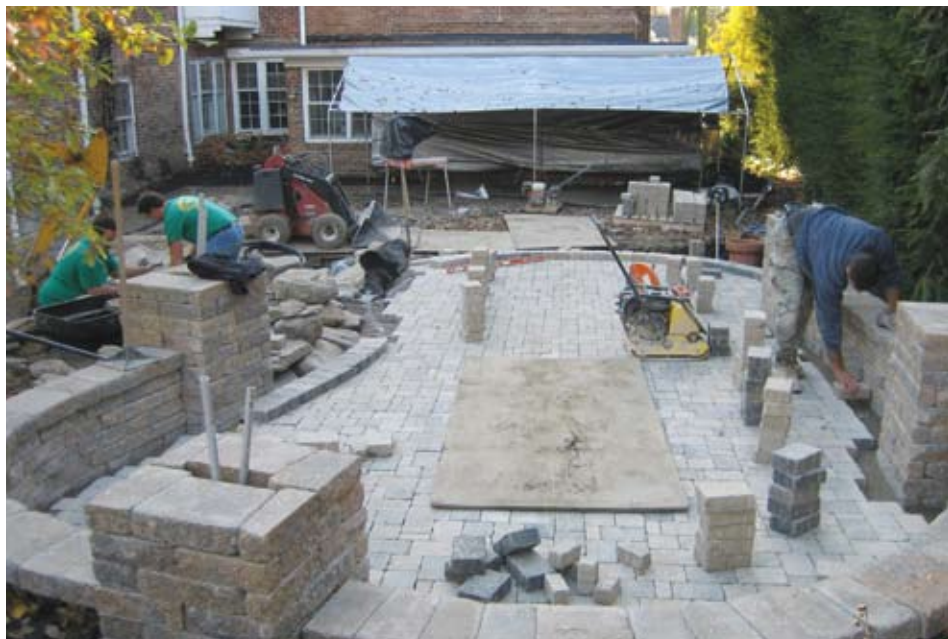
Special equipment and skilled craftsmanship were necessary to complete the site work and installation of this custom patio, retaining wall and water feature project.
